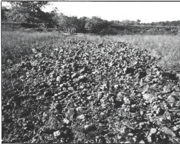
Facing north, this shows the dirt that washed out of the dike.
