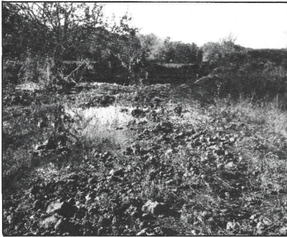
A close look at the broken levee at the Mill Creek River, on Highway 54, more than a mile west of Fort Scott, and three quarters of a mile north.
