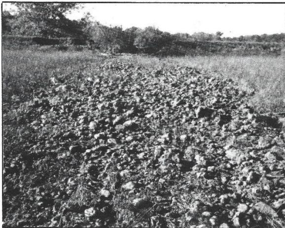
Facing north, this shows the dirt that washed out of the dike.
